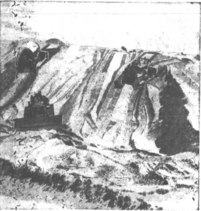
A new pipeline—designed to carry between 300,000 and 450,000 barrels of oil daily—is being pushed across the Saudi Arabian desert. It will run through 1000 miles of sand dunes. Bulldozers carve a path for the 30-inch pipeline in the desert near Ras Tanura.
