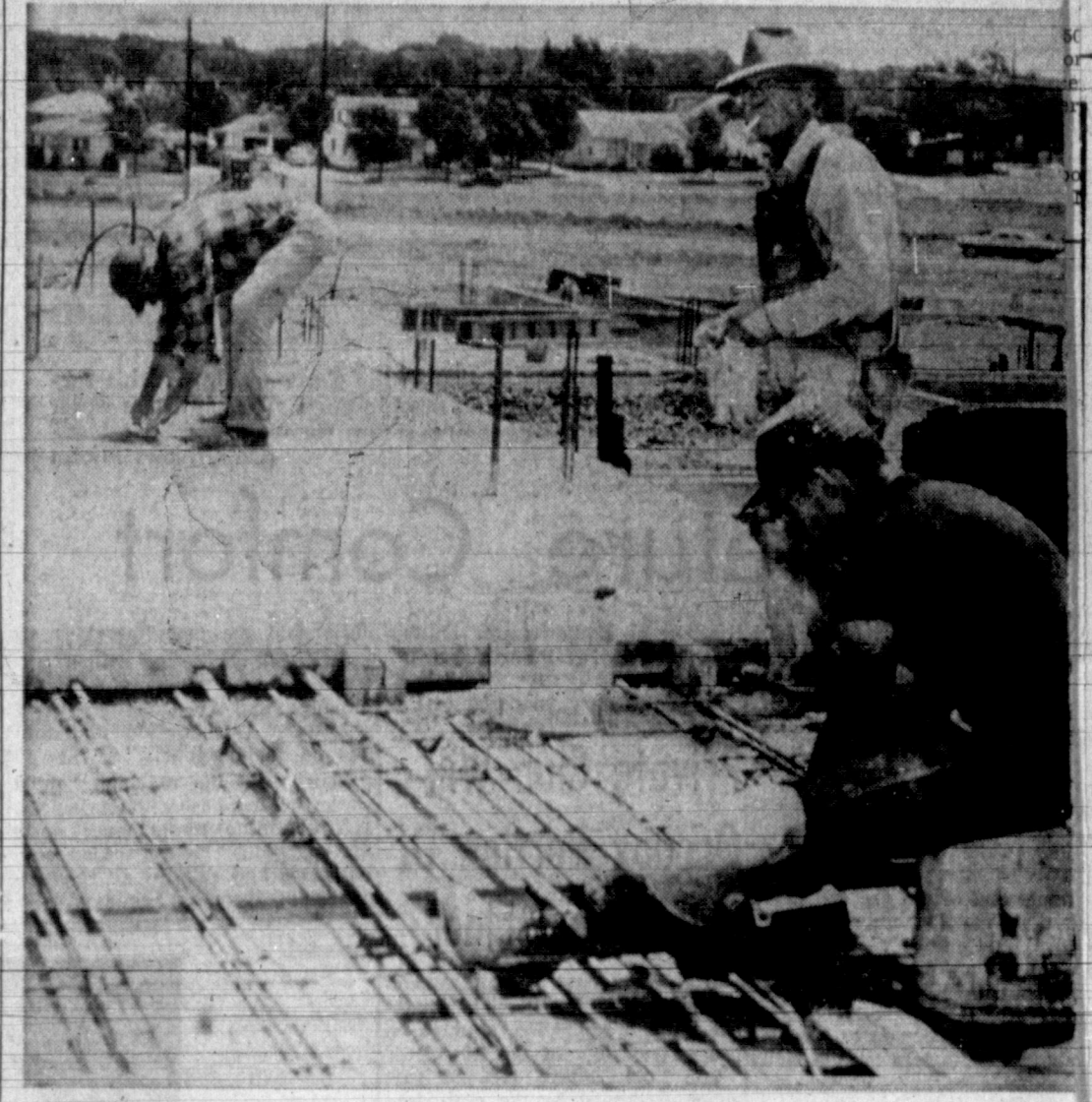
SECOND STORY MEN — Construction progress at the Coronado Inn last June 24 carried quite a different look than the beautiful sight it now presents. Working on the second floor concrete slab are, from left, E. F. Hall and F. B. Hunter, both of Berger and Bill Hunter of Pampa. Progress at that time was right on time, according to construction superintendent Bill Boehme. He called the shot right by stating then that the hotel would be completed January 15. The owners were to accept the hotel from the contractor, Farnsworth and Chambers, Friday. (Daily News Photo)
