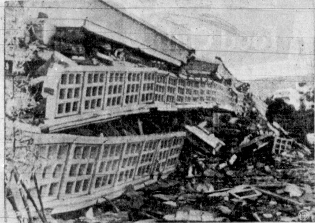
SHATTERED — Rows of shattered windows are all the remains discernible in the wreckage of the multi-storied Saada Hotel in Agadir, Morocco, after the building collapsed in the earthquake that hit the city Tuesday. An estimated 3,000 persons died in the disaster.
