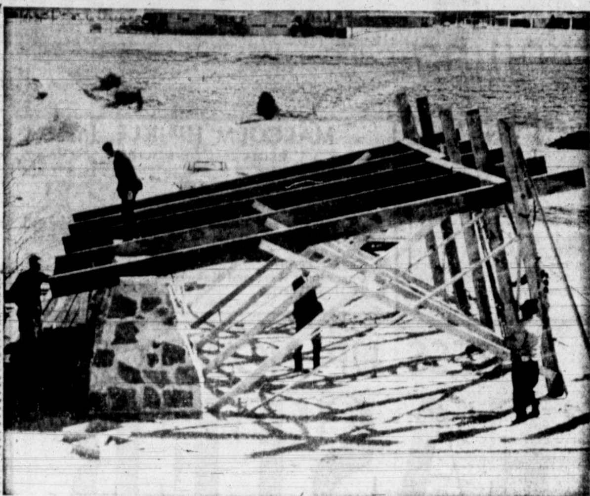
CONSTRUCTION UNDERWAY — The long-awaited construction on the shelter in Aspen Park got underway this week under the direction of the Pampa Garden Club, Junior Chamber of Commerce and the City Park Department. Pictured above inspecting the work to date are Gene Hollar on the roof; Kay Fancher under the beams, Bill Stark in the foreground and two unidentified Park Department employes. Dedication ceremonies are planned for March 30 in the park. (Daily News Photo)
