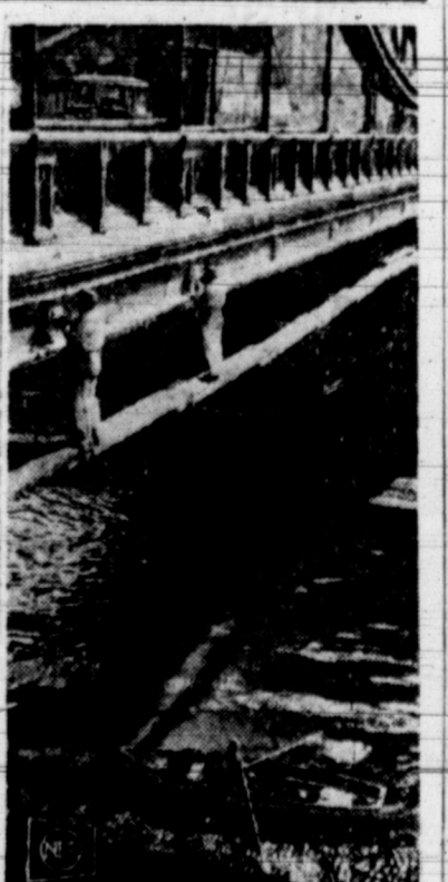
WALK THE PLANK—Men working on the Tower Bridge in London walk the straight and narrow of the planks along side. Man in rowboat, below, stands by just in case.
