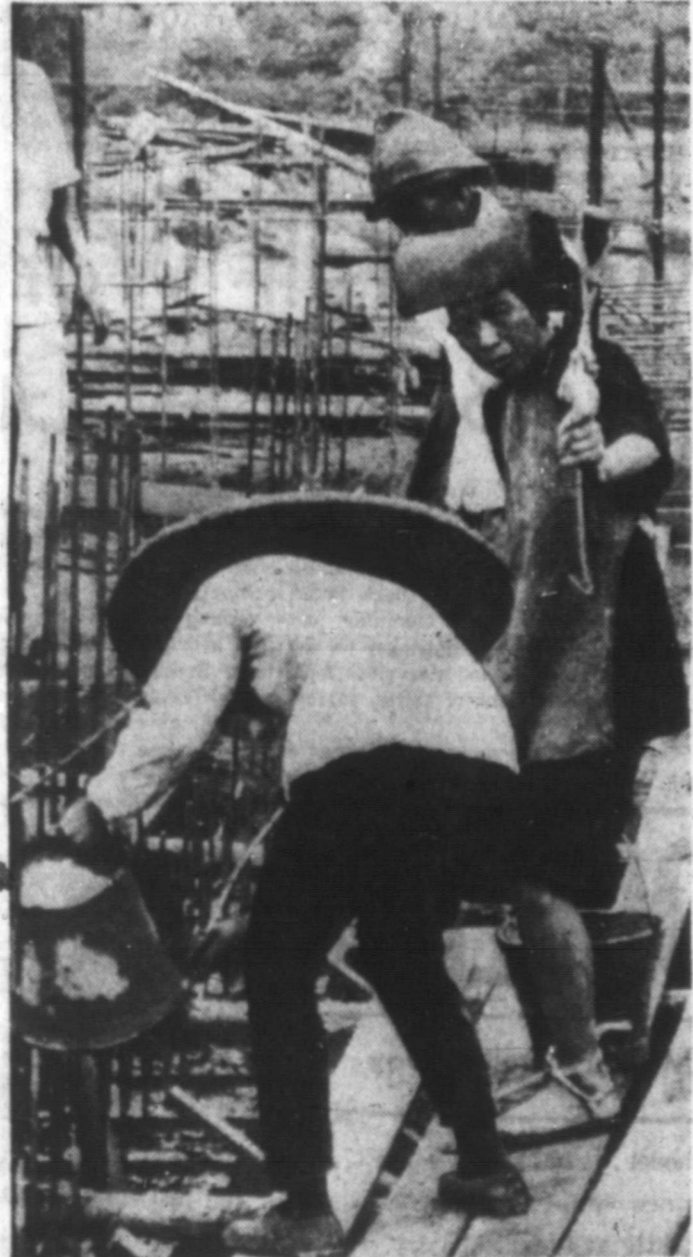
WORKING WOMEN —The Sem swee, the working women of China, are building a housing project in Singapore in a scene from the television show, “The Overseas Chinese.” The Sem swee, mostly from the Canton area, never-marry and usually work on heavy construction in this area.
