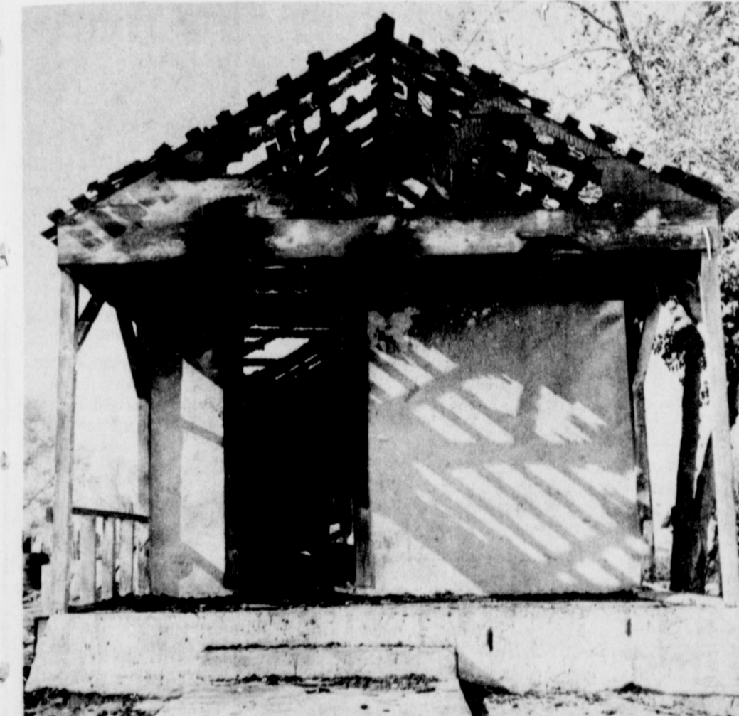
FIRE DAMAGES BUILDING...This building on the west end of North Chicago Street in Muleshoe was the scene of a damaging fire Wednesday night. Three units of the Bailey County Volunteer Fire Department were called to the scene at approximately 10:30 p.m. The contents were estimated to be a total loss and the building extensively damaged by the fire.
