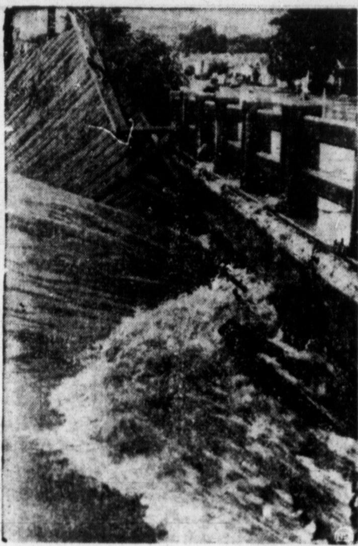
BRIDGE UPROOTED —A two-inch rain in three hours caused flash flooding in San Antonio. The swirling waters of flooding creeks uprooted a wooden bridge and jammed it under a concrete span at Cincinnati and Martinez creeks. Hundreds of motorists were stranded by the high water.
