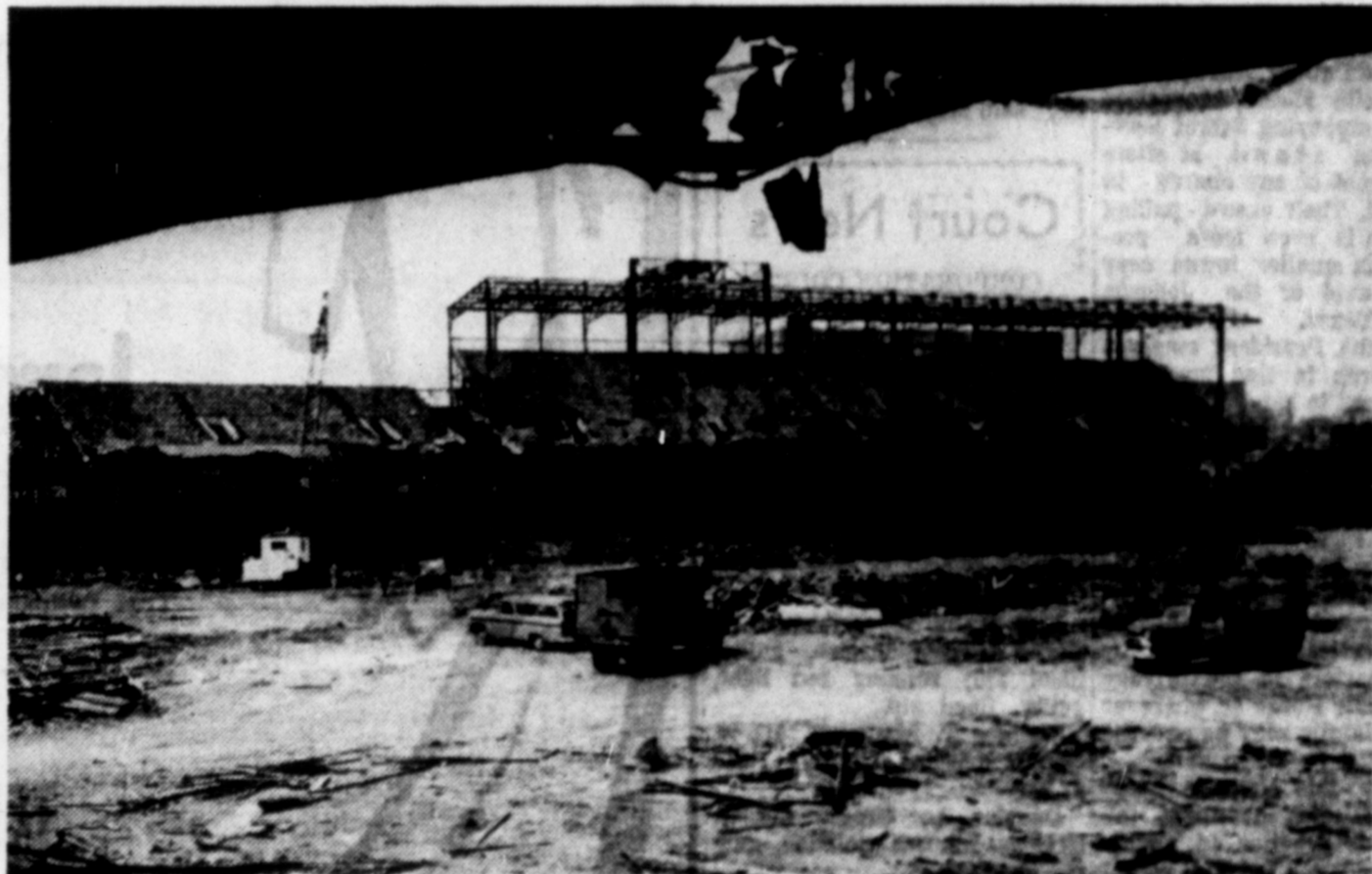
PROGRESS IN WASHINGTON —Fans once came to Washington's Griffith Stadium to root for the baseball Senators and football Redskins, but the only people who come to the old stadium these days are wreckers. Built at the turn of the century, the ancient sports spot is being torn down to expand Howard University.
