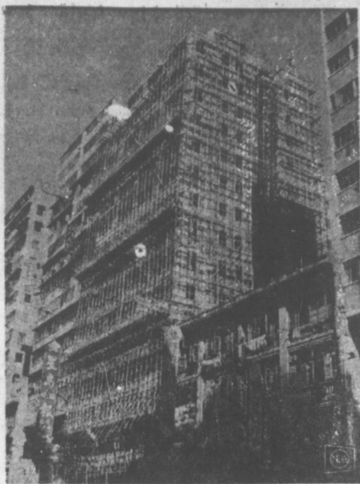
BAMBOO PREFERRED —Steel may be the material for heavy-duty construction in the West, but in the Orient the ancient bamboo is still preferred even for many modern tasks. This new building rising in Hong Kong is festooned with scaffolding built completely of bamboo, instead of the maze of steel pipes usual in the West. Experience has shown that bamboo scaffolding, constructed without nails or metal support, is actually stronger and more stable than similar steel structures.
