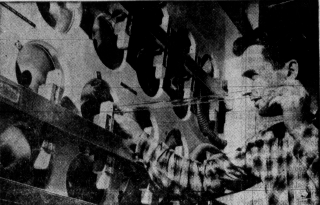
AIR GETS 'SCRUBBED' in Minneapolis' North Memorial hospital, which claims the cleanest air in the country. With air pollution a growing problem in the U.S., this system by Honeywell, Inc., utilizes special filters, plus ultraviolet lamps to kill germs and activated charcoal to eliminate odors. Corkscrew-shaped baffles swirl air around the tubes for a complete ultraviolet cleaning. One of the lamps is being installed here by an attendant.
