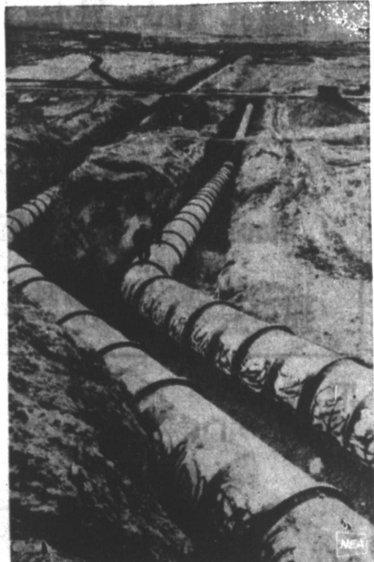
WORKERS WALK along huge irrigation pipes in the arid Yavan Valley of the Tadzhik Soviet Socialist Republic, near the Soviet Union's border with Afghanistan. Soviet engineers are channeling water from the Vakhsh River through the mountains to irrigate the region.
