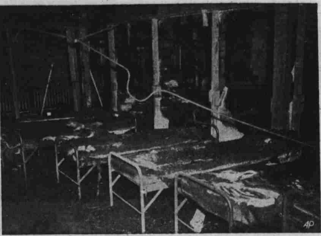
WHERE MEN WERE TRAPPED BY FIRE—This is the charred interior of the sleeping quarters of the Salvation Army men's lodge and mission in the second story of a Dallas building where ten were fatally burned and several others seriously burned in a fire.
