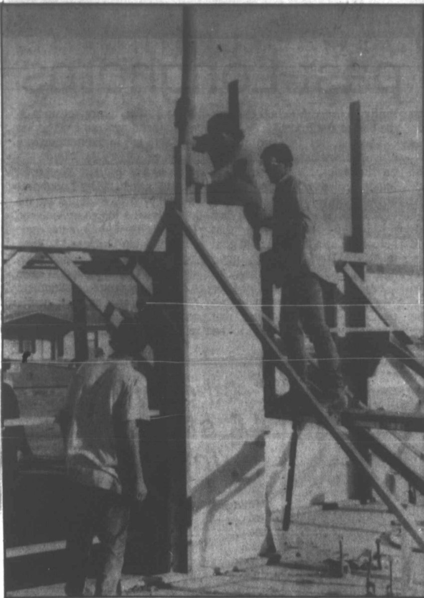
Ernie Casados, center, holds a tube for pouring concrete between wall forms as Carl Whinery, left, and Brandon Kitchens looks on during construction of a house in the Frasier Estates east of Pampa off Highway 60. (Pampa News photo)
