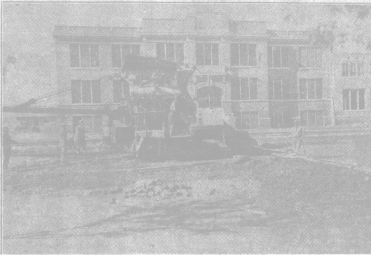
This model 27-E Rex Mixer is the largest used in either road or street paving. Finding enough trucks to feed it is the main difficulty.
