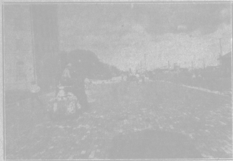
A bad brick is sure to show up under this 5-ton roller used by Stuckey Construction company. Rollers half this weight are often used elsewhere.
