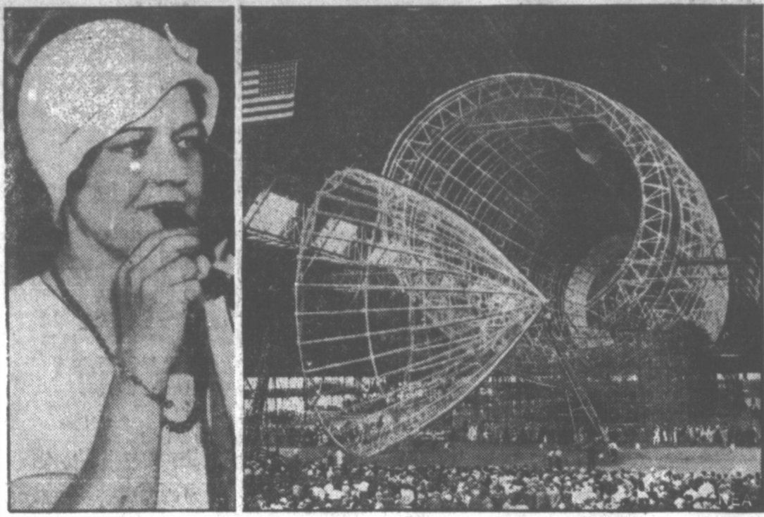
The U. S. navy's mammoth new airship, the U. S. S. Macon, entered the final stages of construction at the Goodyear-Zeppelin dock in Akron, O., when its 75-foot bow was lifted into place with elaborate ceremonies. The larger photo above depicts the scene as Miss Susan Myrick, left, of Macon, Ga., blew a whistle to start cranes hoisting the airship's nose into place.
