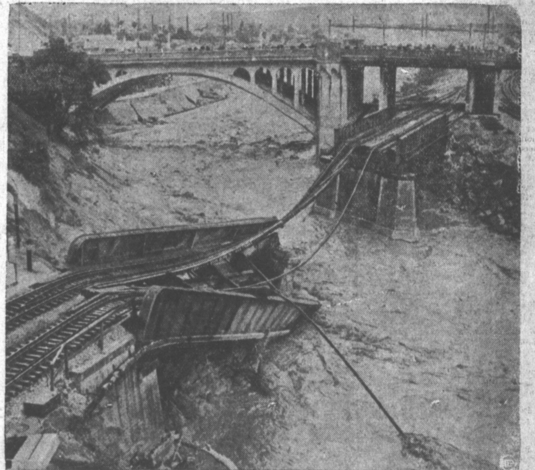
Once stout enough to support a train but now torn literally to ribbons by raging flood waters this steel railway span was washed from its base and deposited partially in the bed of the Los Angeles river.
