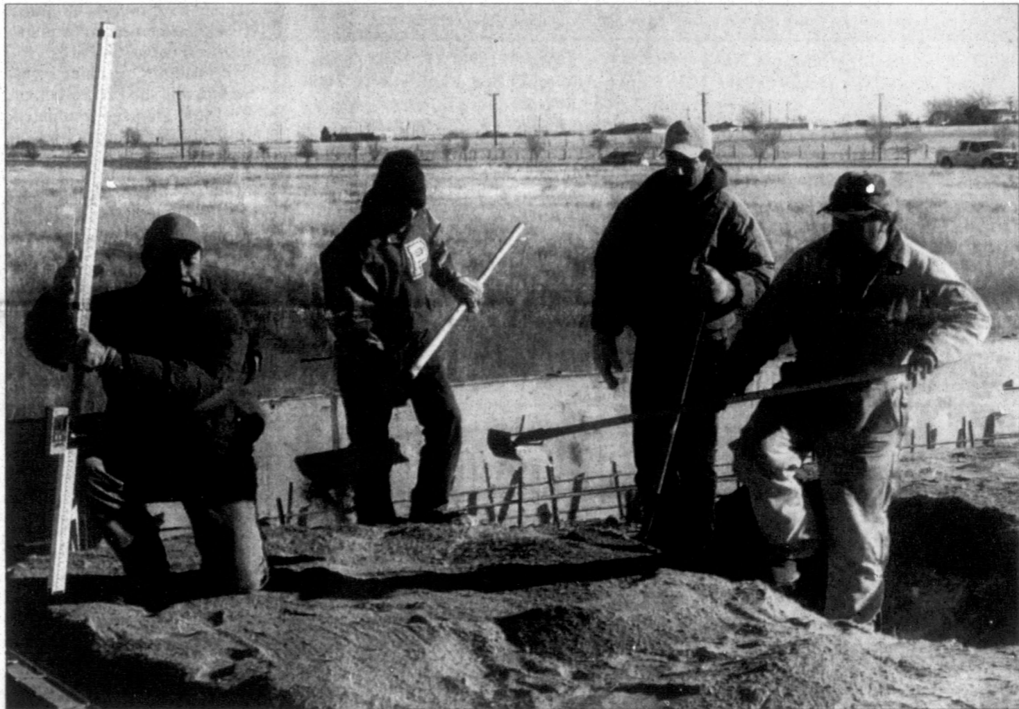
A work crew prepares the ground before pouring the foundation for a new Holiday Inn Express, under construction north of Pampa Regional Medical Center on Highway 70. From left are Jesus Jimenez, Alberto Guerrero, Arturo Barrera and Ruben Becerril. The hotel's owners, Dipak and Sangita Patel of Amarillo, said in an April 9 interview that they plan to have the structure completed and ready for business in May. The Patels also own a Comfort Inn and a Country Inn and Suites in Amarillo.
