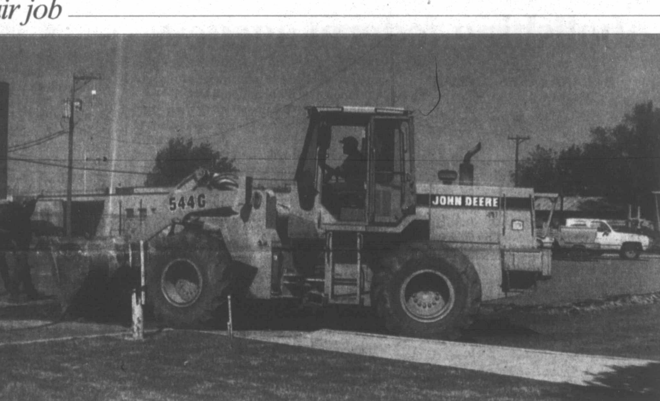
Employees of G. W. James Inc. making repairs to the parking lot at the Pampa Community Building this morning included, from left, Rick Caughey, Junior Hartley and Nacho Vargas, who operated a front end loader.
