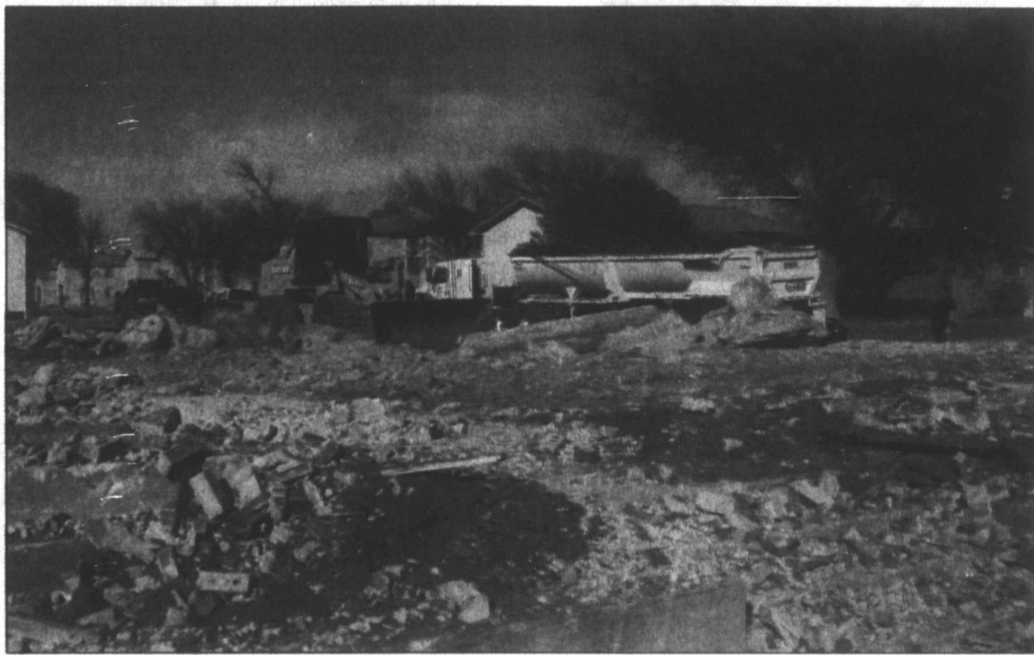
Demolition is under way by R and R Ditching Co. from Lubbock at the corner of Hobart and Kentucky streets, making way for a new CVS Pharmacy. Norman House, right, waits for his dump truck to be filled by the front end loader. Valerie Walker, one of the dump truck drivers, said that work is scheduled to take about three weeks.
