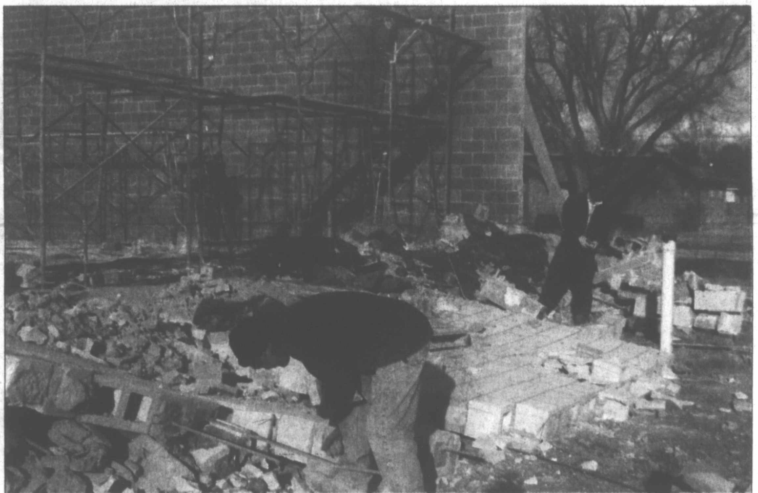
The south wall of the new CVS building came tumbling down Thursday, but it was intentional. Ramone Ramirez, left, and Juan Ramos from Bobby Lee Construction in Dallas picked up the pieces to be hauled off. Ramirez said the concrete did not set correctly so they had to knock down the wall and start over. The outside shell should be complete in 4 to 5 days.
