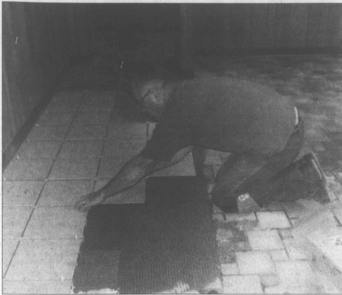
Contractor Louis Austin from One Stop Flooring lays new tile today in the public area of the Chamber of Commerce building after the carpet was removed.
