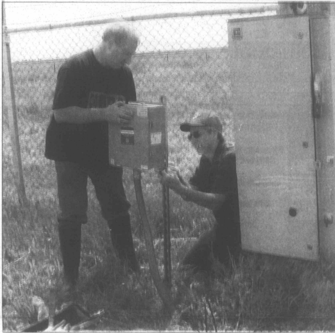
Pampa News photo by MARILYN POWERS Sam Johnson, left, president of Johnson-Aire, Inc., and Wayne Johnson install a Circuit Master at a city of Pampa water well off County Road 7 1/2 south of McCullough Avenue. The city is having the devices placed on all working city water wells in order to save energy, reduce wear and tear on electric motors and protect against power surges and spikes.
