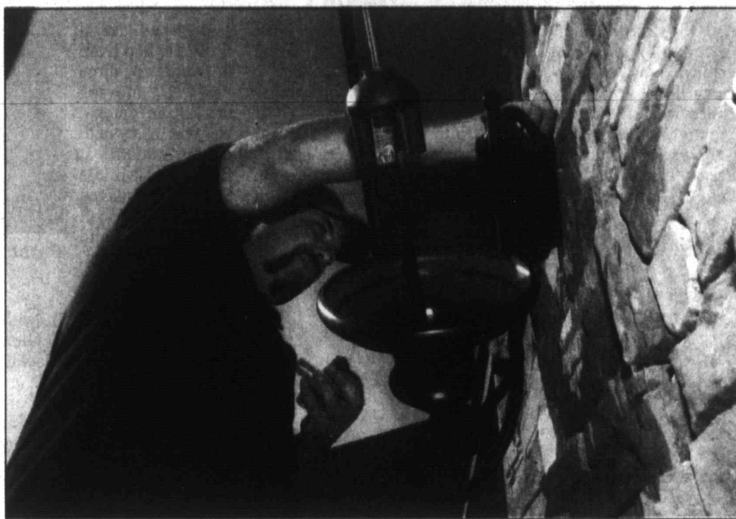
Pampa News photo by DAVID BOWSER Dave Davis, an electrician with Mac Supply, installs lights at a new home being built by Giles Custom Homes. Of the six new homes they plan, five are under construction. Pampa's population is growing.
