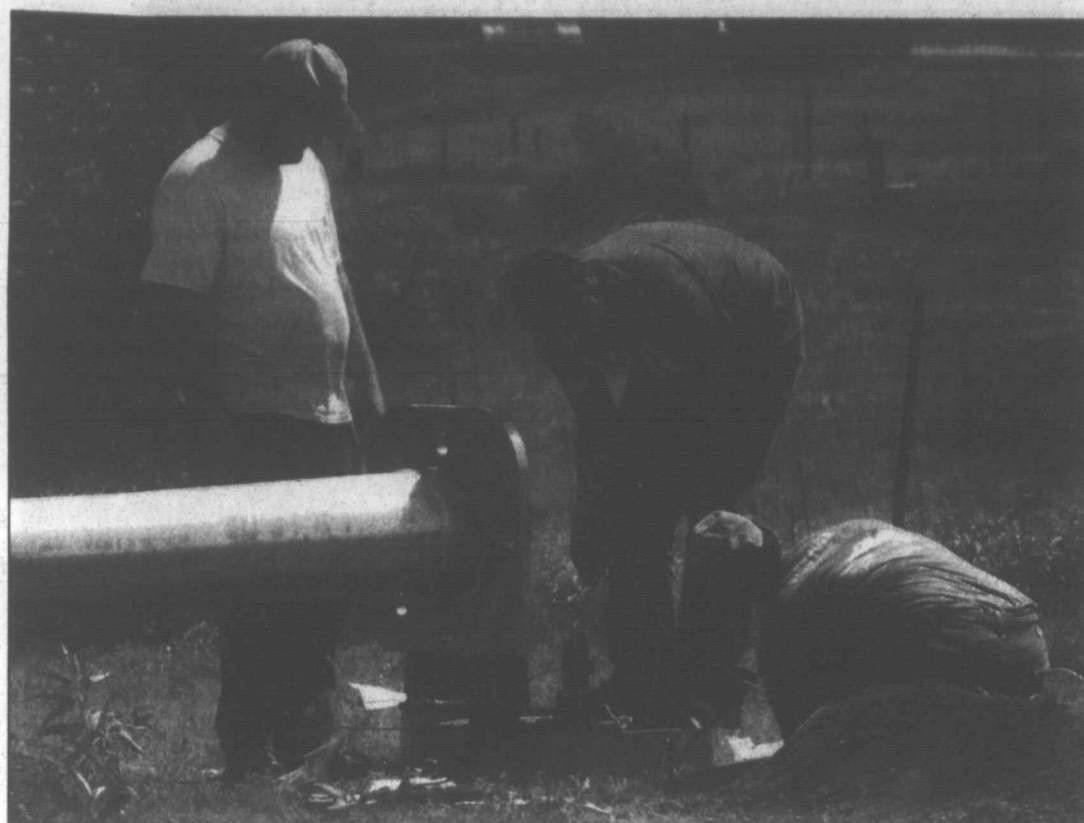
staff photo/R.Stennett Cesar Ramos (right), Windworks Energy employee, installs the residential wind generator at the Davis home with co-worker Felipe Hernandez (second from the right) and Pampa worker Toby Meeks (left). They used Mac Supply for electrical supply in the project.
