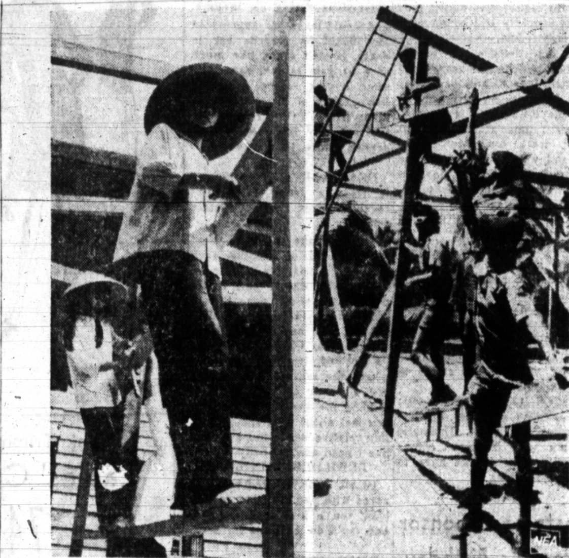
HIGH SCHOOL GIRLS, left, and Boy Scouts in South Vietnam help build housing for families made homeless by Communist attacks on Saigon. The Agency for International Development is providing shelter for nearly two million refugees. Allied troops have been finding arms caches supposedly being prepared for a new assault on Saigon.
