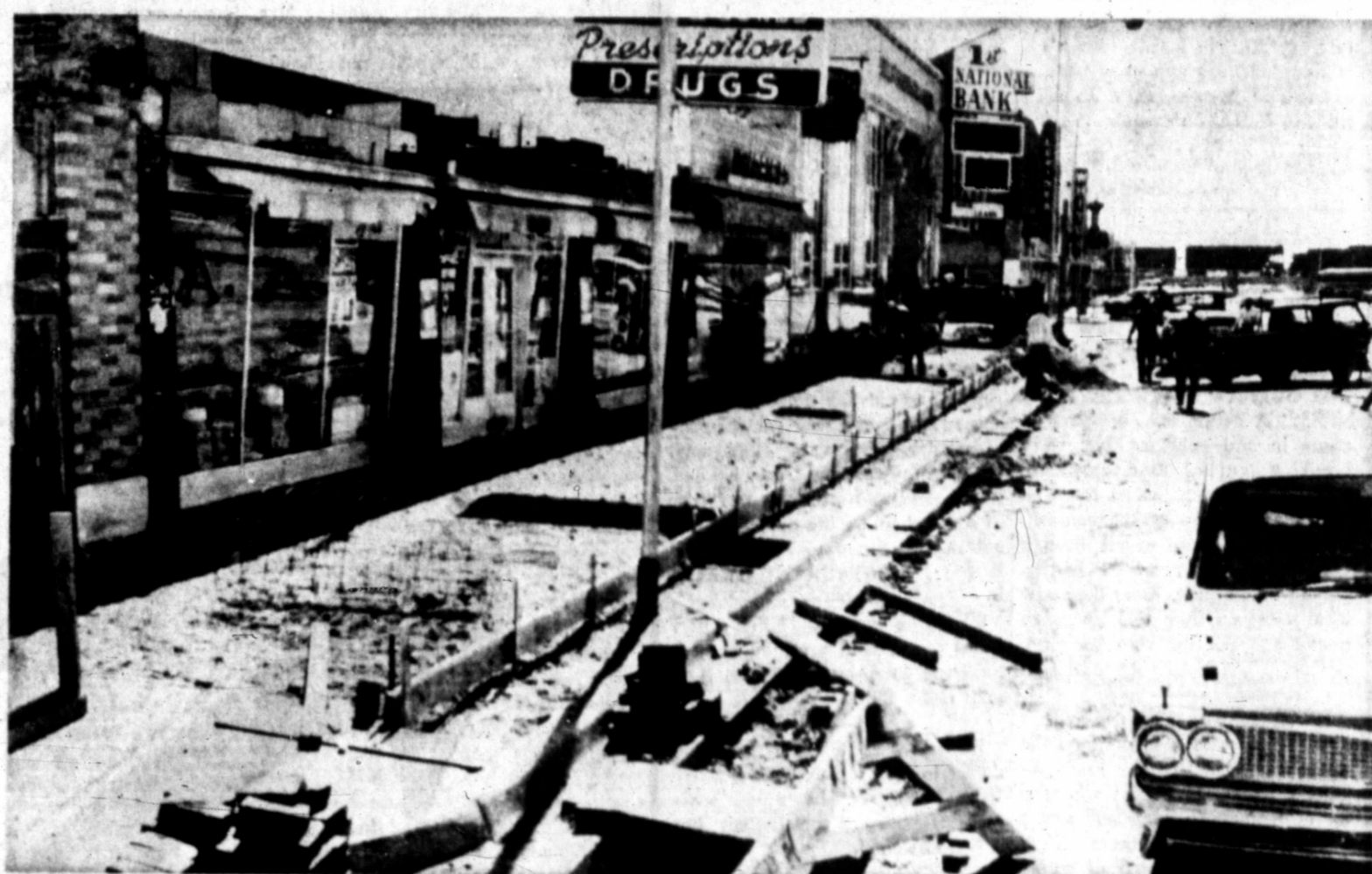
NEW CURBS FOR CUYLER — New curbs and sidewalks to be constructed in the 100 block of N. Cuyler this week. The new curbs will permit parking without scraping or denting the bumpers of cars. Construction is proceeding rapidly and should be completed shortly. (Daily News Photo)
