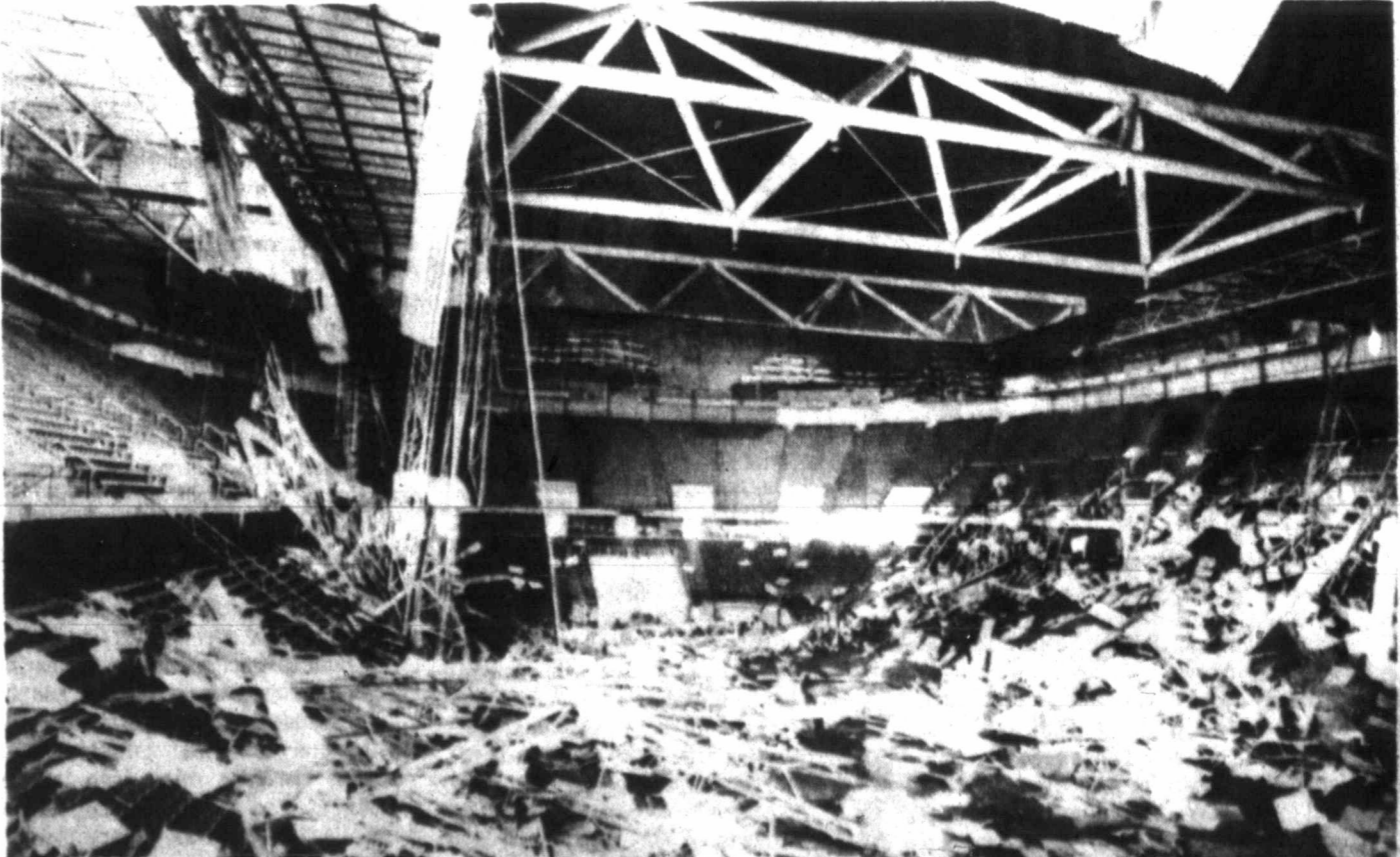
NEARLY ALL of the roof of the 17,000-seat Kemper Arena in downtown Kansas City collapsed Monday night during a severe thunderstorm that dumped three inches of rain on the area in less than an hour and was
