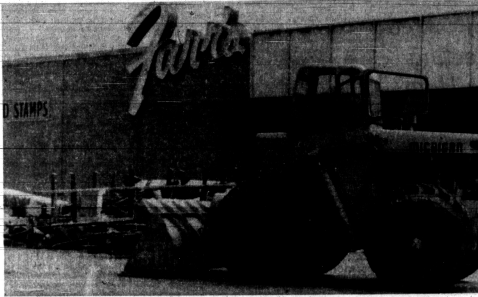
A BULLDOZER in a grocery store has been an unaccustomed sight for the past week and a half as workmen removed fire-blackened merchandise, destroyed in the half-million dollar fire which ravaged Purr's Food Store, 1420 N. Hobart in the early morning hours of Sept. 5. Complete leveling of the building is expected to be complete by Friday. (Staff Photo)
