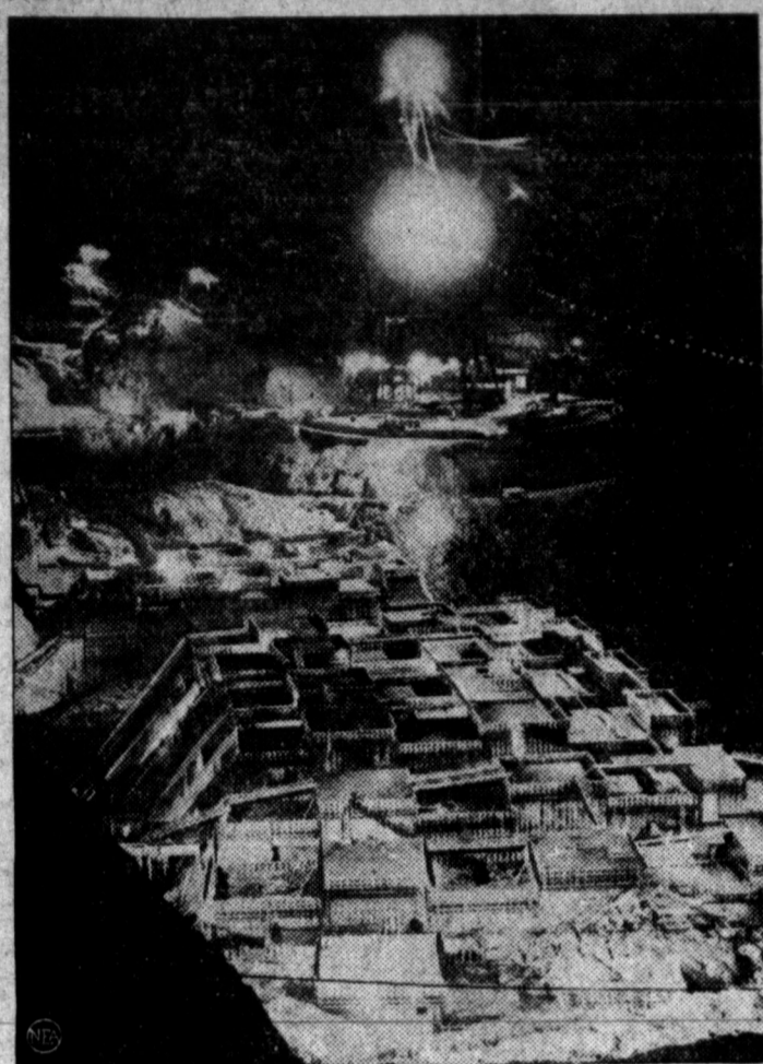
Striking picture shows construction on Shasta Dam in California, where work continues 24 hours a day.
