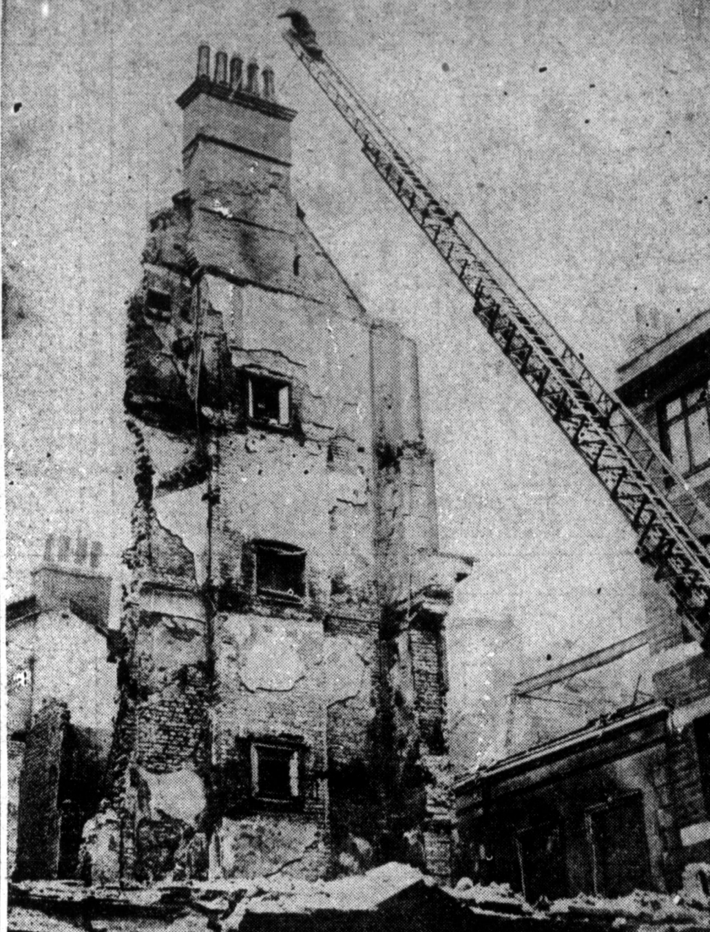
Spectacular picture—illustrates one of tough jobs left for Londoners after the bombers have gone. A demolition worker goes way up there on a giant crane to fix steel cables to the wall of what was an office building before remains are pulled down.
