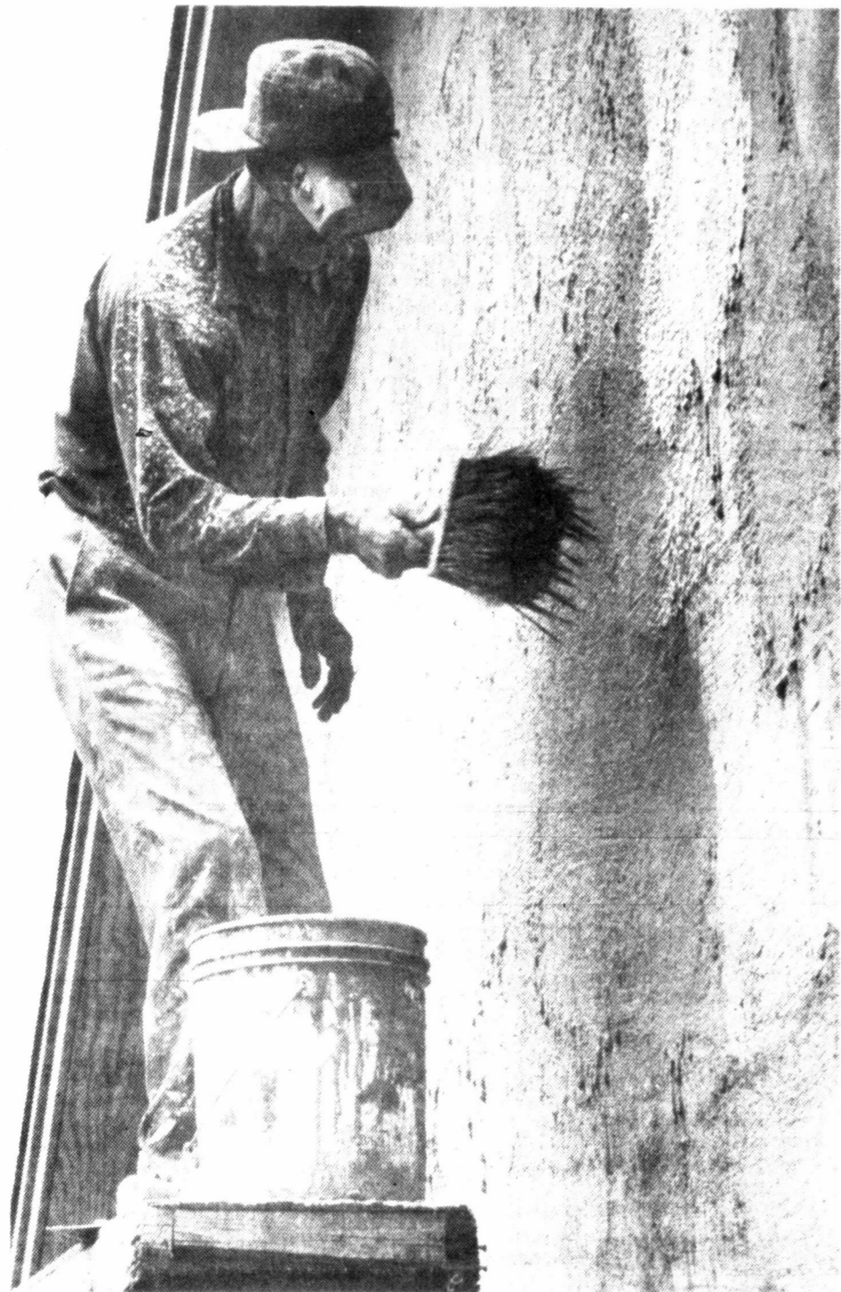
SPRING CLEANING for Harley Smith of 1210 S. Hobart included renovating his home, inside and out. The clouds today did not deter Smith who continued putting stucco on the exterior of his house. Clouds and possible rain showers are forecast for Tuesday. (Staff Photo by Skyler Chapman)
