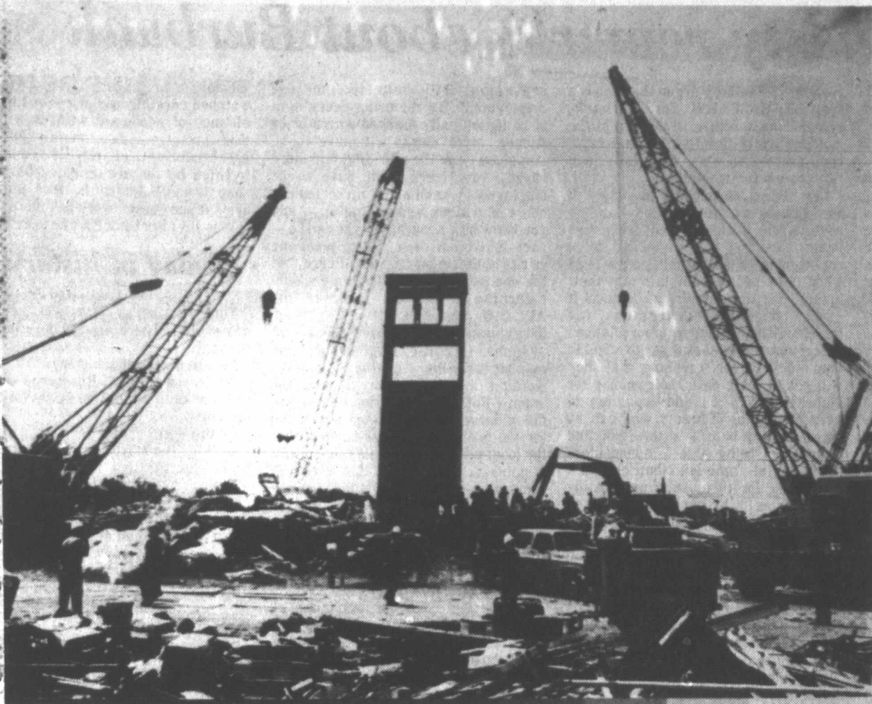
COLLAPSED CONDOMINIUM. Cranes and volunteer workers continue the task of removing the last of the debris from a collapsed Harbour Cay Condo at Cocoa Beach, Fla. The only thing that was left standing was the elevator shaft. Collapse of the condominium as it was under construction killed a score of workers. The last body of the known missing was recovered Sunday. (AP Lazerphoto)
