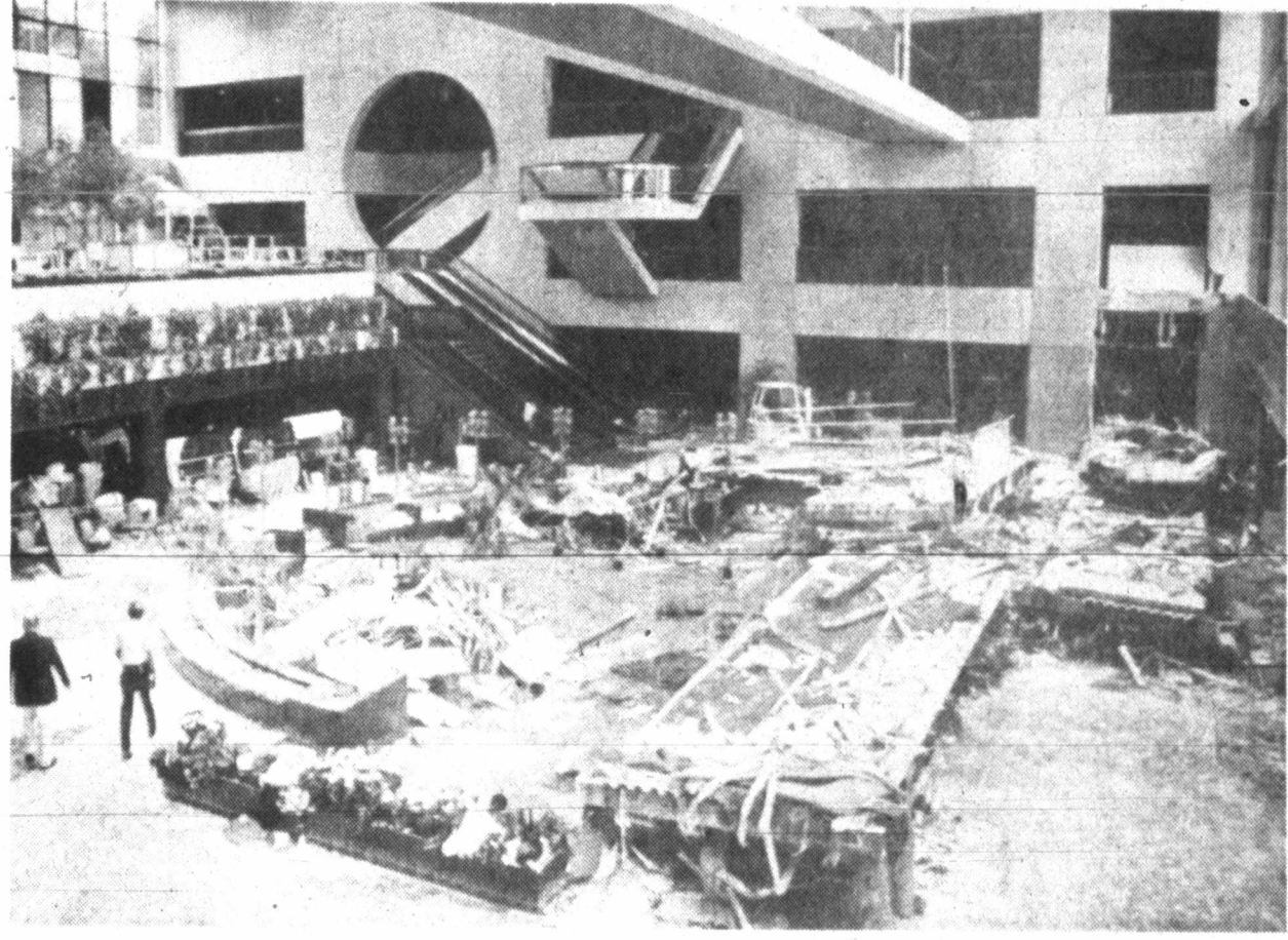
WHERE CATWALKS TORE LOOSE. A police officer and three unidentified people stand near the third floor catwalk above the lobby of Kansas City's Hyatt Regency Hotel Sunday. The fourth and second floor catwalks that
