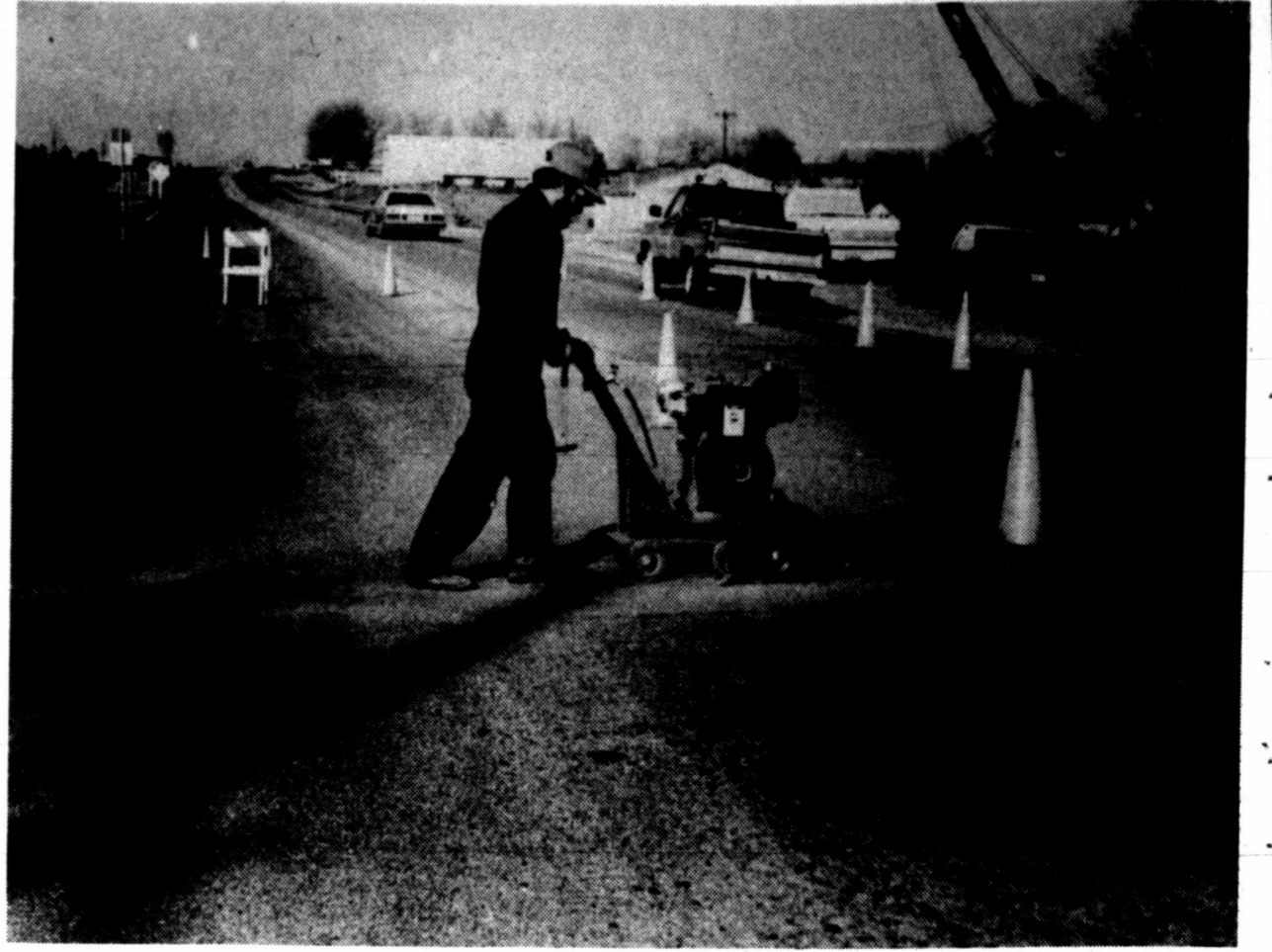
TRAFFIC LIGHT INSTALLATION. John Dunn of Pampa, an employee of Ray Electric, uses a gasoline-powered saw to cut the pavement at the intersection of West Alcock (Highway 152) and Price Road (Farm to Market Road 282) in preparation for installation of traffic detector loops for the new traffic lights being installed at the intersection at Pampa's west edge by the Texas Department of Highways. (Staff Photo by John Wolfe)
