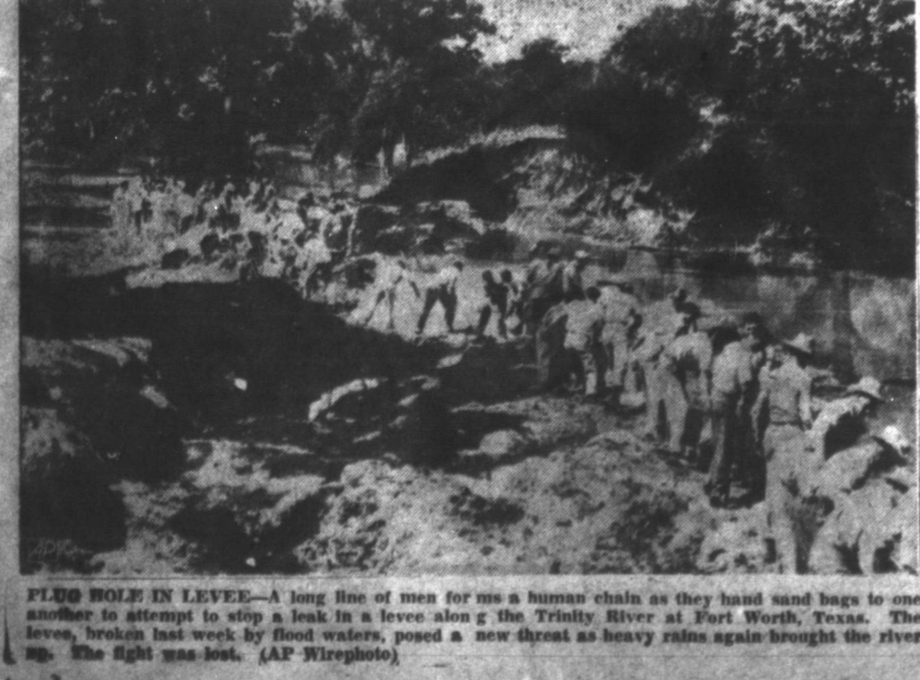
FLUO HOLE IN LEVEE—A long line of men forms a human chain as they haul sand bags to one another to attempt to stop a leak in a levee along the Trinity River at Fort Worth, Texas.
