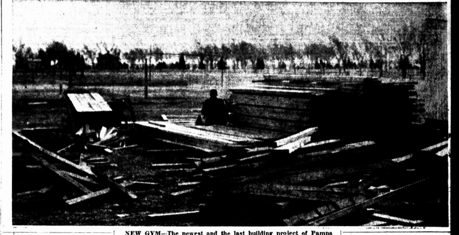
NEW GYM—The newest and the last building project of Pampa schools is underway. Work has started on the field house and vocational classrooms. The building will be set up just north of the old high school gymnasium near Harvester Park. The field house will face the stadium. James T. Taylor and Sons of Fort Worth are the contractors. The building will house wood-working shops and vocational agriculture classrooms along with storerooms for football and basketball equipment, and shower rooms. Permanent bleachers, will be built over the classroom for basketball spectators. (News Photo and Engraving)
