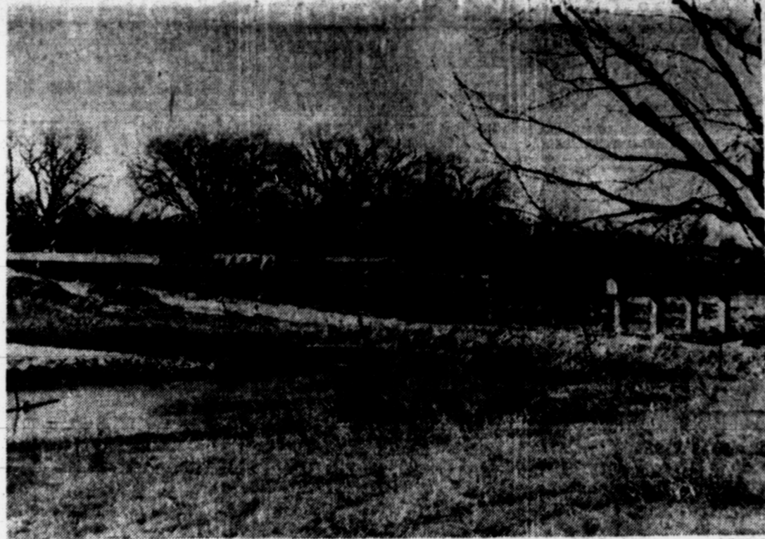
SPANNING THE INVITING waters of Chicken Creek, along State Highway 70 between Pampa and Perryton, this steel reinforced, concrete bridge slowly nears completion. The decking, now being poured, is divided into 12 concrete slabs 25 feet long by a 26 foot roadway. Only five of the slabs are in place here, but if the weather warms up the remaining seven should go down in a hurry, engineering officials hope. (News Photo and Engraving)
