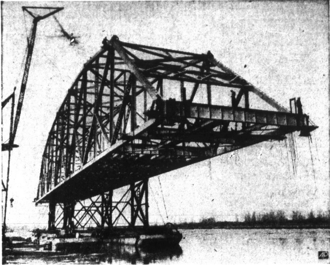
BRIDGE SPAN AT REST — Bridge span for a highway over the Calumet river in Chicago rests on a barge as preparations are made for floating it into place.
