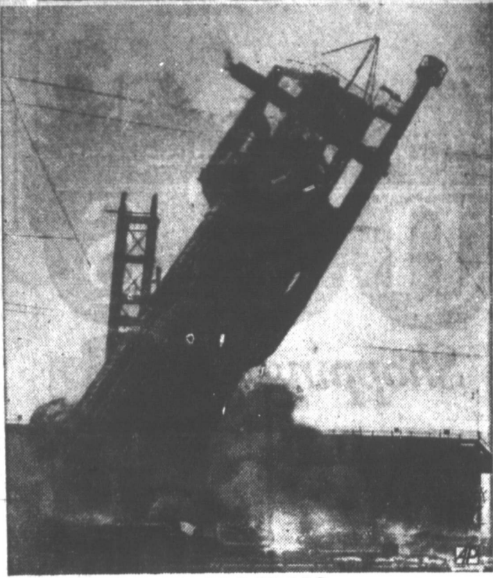
CASUALTY OF PROGRESS —Dynamite and a steel cable attached to a locomotive send this blast furnace toppling during renovation of the Minnequa Works in Pueblo, Colo.
