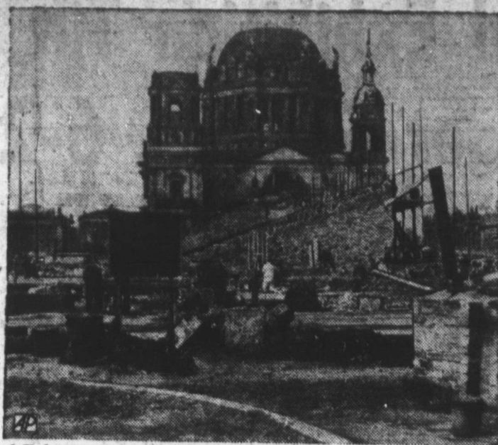
STAND REPLACES CASTLE — Workmen construct a reviewing stand for a Moscow-style May Day parade in E. Berlin on site formerly occupied by famous Hohenzollern Castle.
