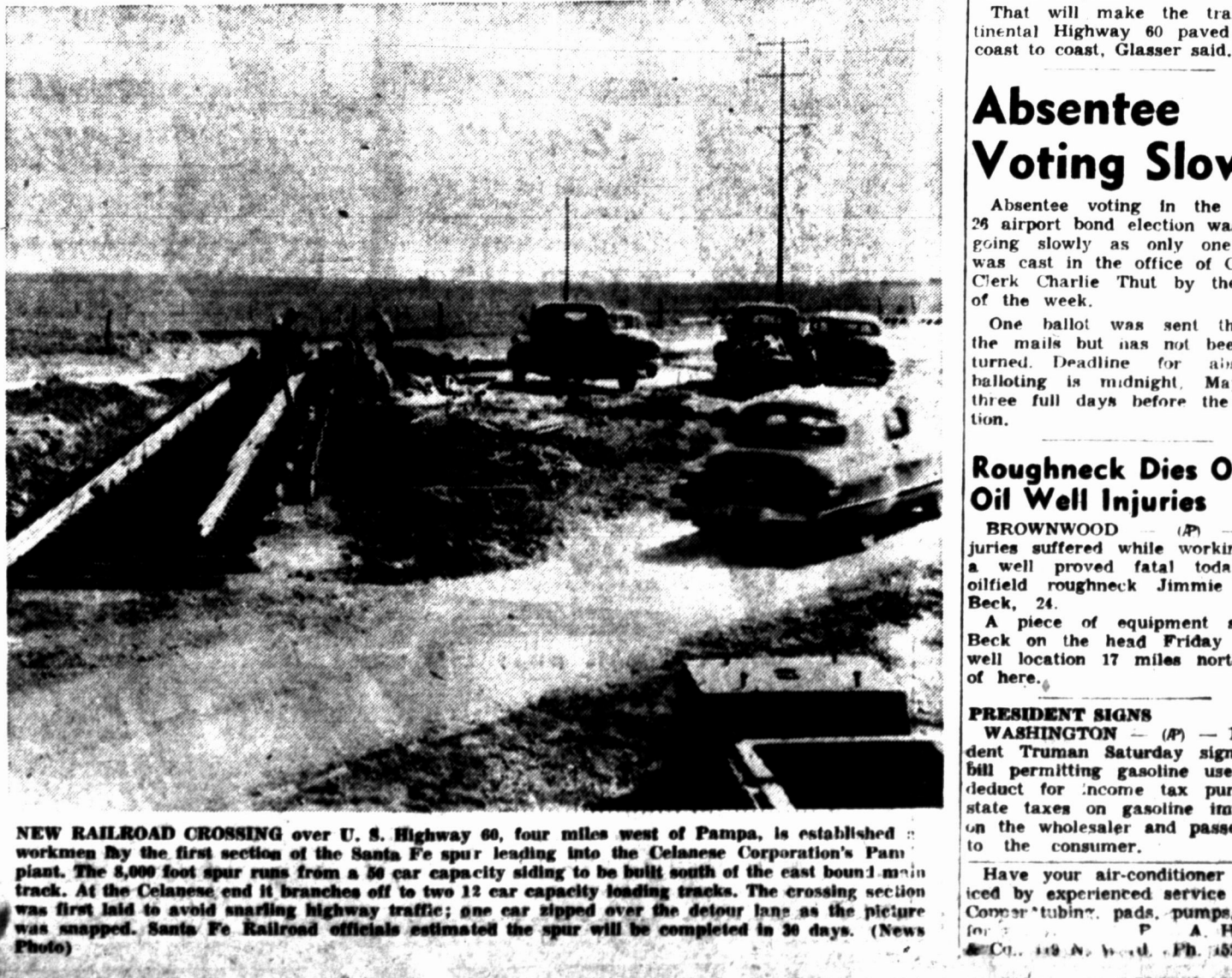
NEW RAILROAD CROSSING over U. S. Highway 60, four miles west of Pampa, is established by the first section of the Santa Fe spur leading into the Celanese Corporation's Pampa plant. The 4,000 foot spur runs from a 39 car capacity siding to the east bound main track. At the Celanese, it branches off to two 12 car capacity loading tracks. The crossing section was first laid to avoid snarling highway traffic; one car slipped over the detour loop as the picture was snapped. Santa Fe Railroad officials estimate the spur will be completed in 30 days. (News Photo)
