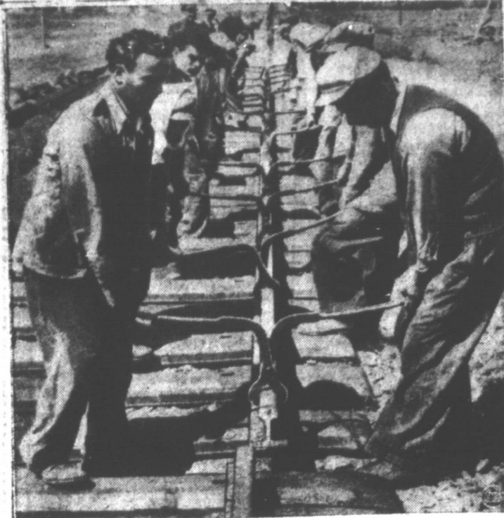
GREECE SNAPS BACK —With hand tools and plenty of elbow grease, workers at Salonika, Greece, put a newly-arrived steel rail into place to repair one of their many war-damaged lines. A full consignment of rails shipped from Western Europe was unloaded and set into place in one day, dramatizing the return to pre-war efficiency of Greek railroads.
