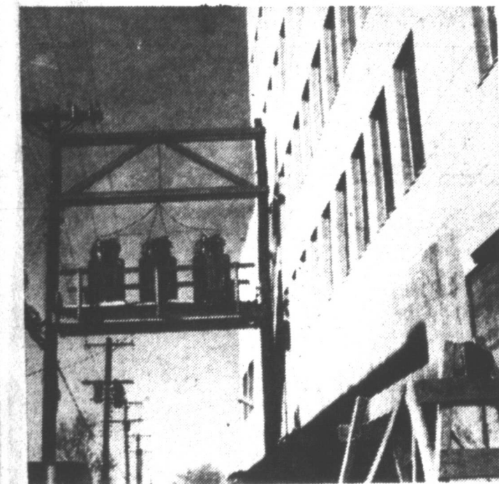
TOP OF THE BUILDING — This photograph shows a view of transformers that reduced high voltage for all electricity in the building. In January, 1951, the office building was being finished up. (E. L. Campbell Photo)
