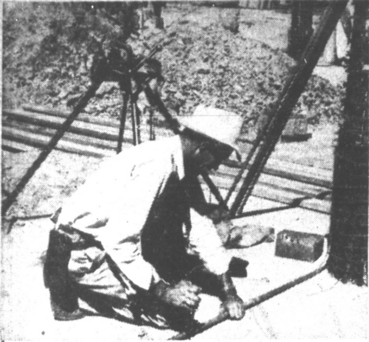
CARL SHARP, electrical foreman, is pictured at work in the basement in September, 1949. The work had been going on six months at this time. (E. L. Campbell Photo)
