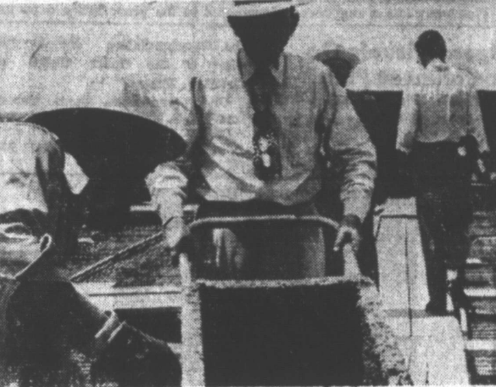
HUGHES, THE BUILDER — Dick Hughes tries his hand at pouring cement as a worker in the foreground tills the cart. In the right background, Hughes' son, Richard, is walking away. (Photo by E. L. Campbell)
