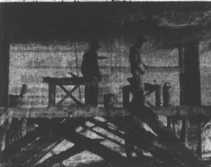
LAST PLASTER in the Hughes Building was done March 29, 1951, in the drug store occupying the first floor of the building. Here men work on the ceiling. Wood frames in the foreground occupy the spot now held by modern soda fountains. (E. L. Campbell Photo)
