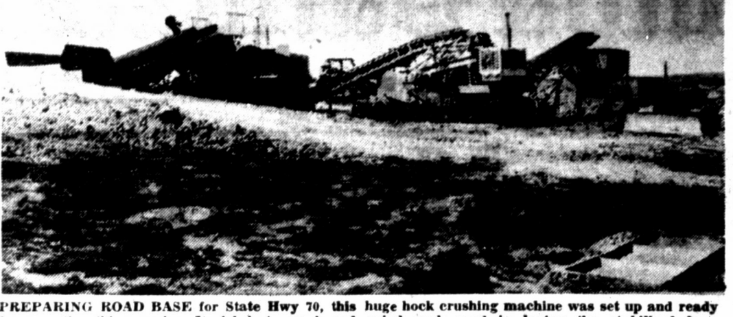
PREPARING ROAD BASE for State Hwy 70, this huge rock crushing machine was set up and ready for operation this morning. Its job is to crush and grind rock used in laying the stabilized base for the highway. The machine pictured above is reported to have a production capacity of 8000 cubic yards of crushed base rock per 16-hour day. The average crusher produces 2000 cubic yards of rock per 10-hour day. Actual production will start tomorrow after road graders have completed rebuilding sub-grades washed out by last week's rains. (New Photo)
