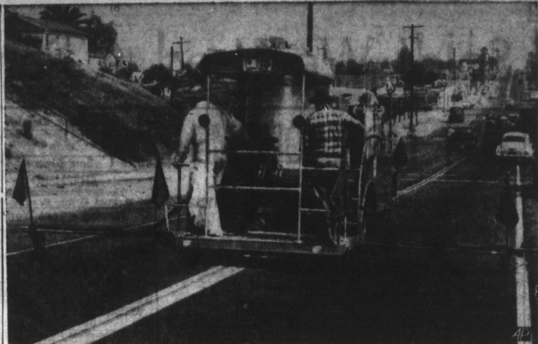
LAYING DOWN THE LINE — Street stringing machine invented by a Tacoma, Wash., policeman, lays down double center line and two outside lines in Los Angeles demonstration.
