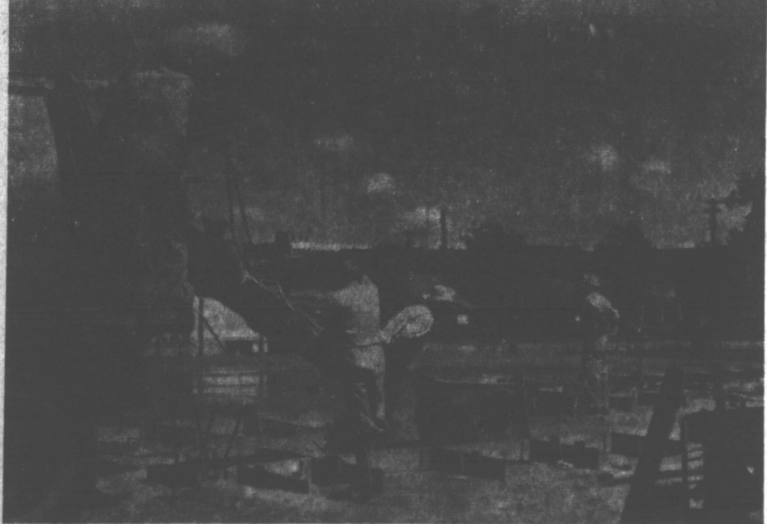
FLOOR SECTIONS POURED — The expensive all-concrete floor for The Pampa Daily News was poured in sections using pre-mixed concrete. Here, workmen are shown pouring a section on the west side of the building located on Atchison at Somerville. (News Photo)
