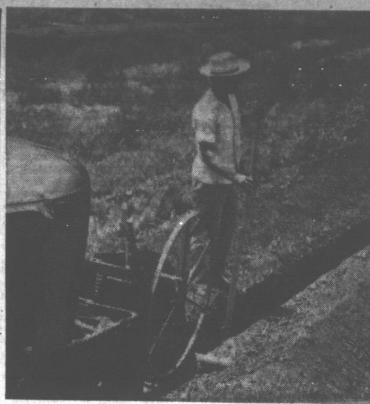
CHECKING DEPTH — A workman, above, helps to check the depth of the foundation trench as The Pampa Daily News began construction on its new plant almost a year ago. (News Photo)
