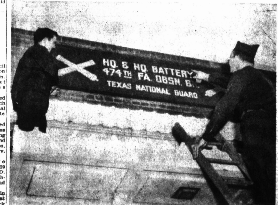
FINISHING TOUCHES — Two members of the local National Guard unit complete raising a sign over the old Cabot Carbon Co. offices on W. Brown. In charge of the erection are Warrant Officer William Leonard, right, and Pvt. Wesley Langhaug. Negotiations for occupancy by the National Guard of the building were completed Dec. 21 after a fire destroyed the Pampa armory Nov. 20. (News Photo)
