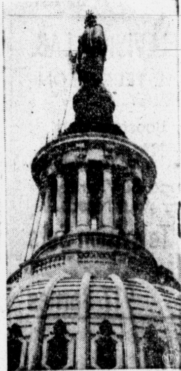
FIXING HER CROWN —The Statue of Freedom, atop the U. S. Capitol in Washington, will have her crown touched up. Steeple-jack Jack Mathis is about to remove platinum lighting arrestors from the crown for replating.
