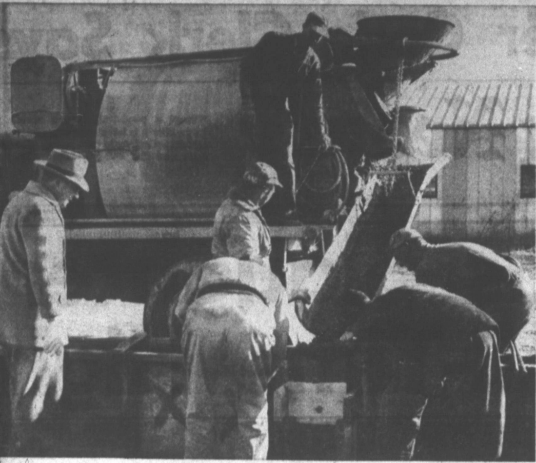
FOUR FOUNDATION — Workmen were busy this morning pouring concrete for the foundation for the four purpose barn at Recreation Park. Pictured above are workmen pouring the footings for the foundation. At the extreme left is Wayland Merriman, engineer for Gray county. Standing, left to right, nearest the truck are J. C. Hutchins, foreman, and Reuben Porter. Nearest the camera, left to right, are Marcus Mata and Claude Adams. Standing on the Trans-Mix Concrete company truck is Jim Kindle of that company. Pouring of the foundation was expected to be completed today. (News Photo)
